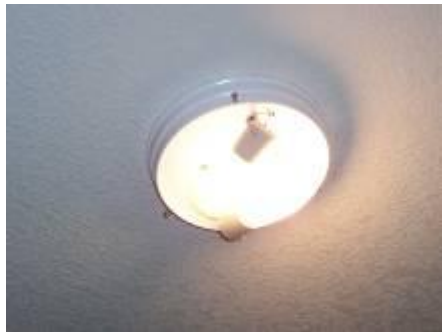
Missing fixture cover
