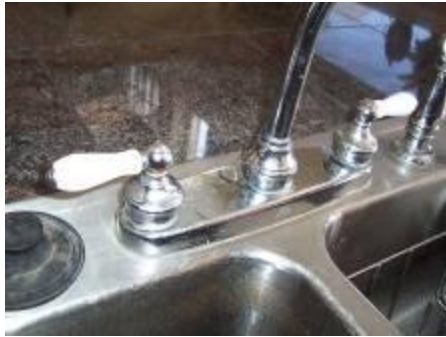
Faucet leaking slightly
