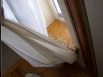
Damaged window trim
