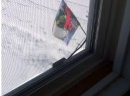
Minor screen damage
