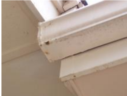
Rust on gutters
