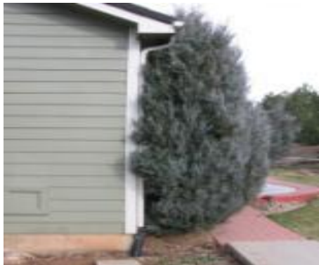
Tree encroachment at rear
