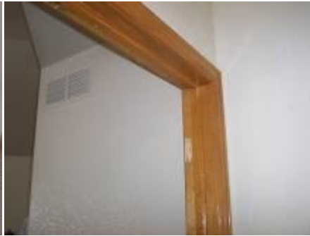
Master bedroom door missing
