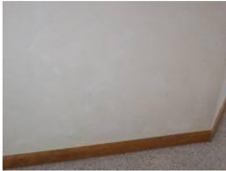
Patching observed in hall
