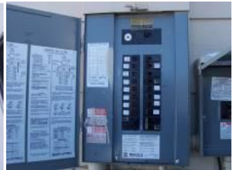
View of main panel
