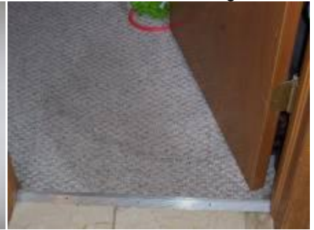
Loose carpet in closet
