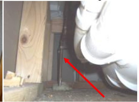
Leak under tub faucet
