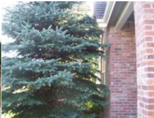
Large tree near foundation at front
