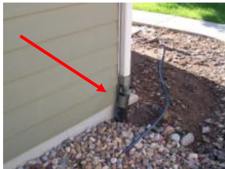
Downspout under grade
