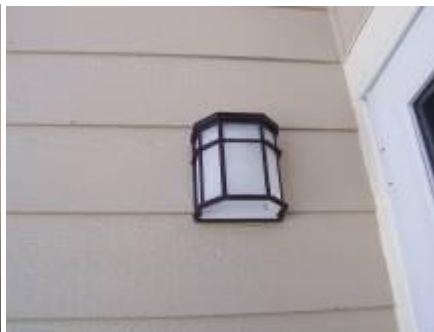
Inoperative porch light
