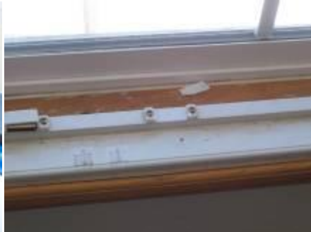
Damaged shutter magnets
